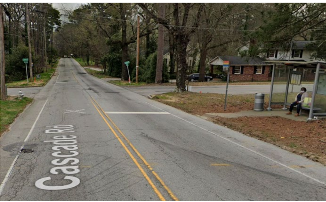
Missing Sidewalk, Crosswalk and ADA Ramps at Cascade Road and Adams Drive & Lynway Lane
