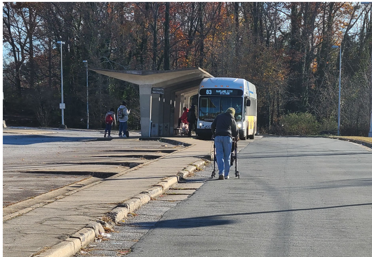
Deteriorating sidewalk and missing ADA Ramps at Barge Road Park and Ride
